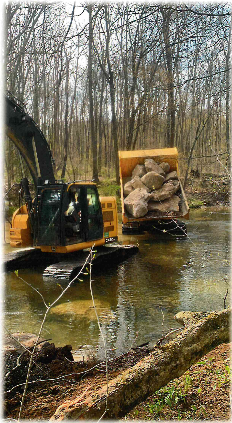
Boulders being placed in the stream for the construction of a rock cross vane.
